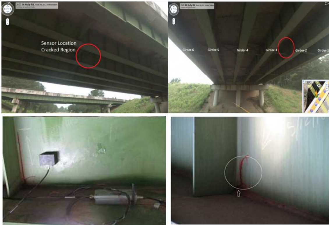
Figure 1.2. Fatigue crack at steel girder in Rock Hill, SC at Intersection I-77/SC901.
